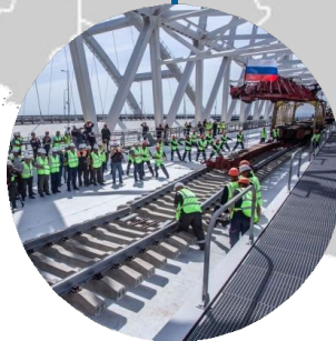
Engineering means of ensuring transport safety during construction of railway tracks to the Kerch Strait crossing point
